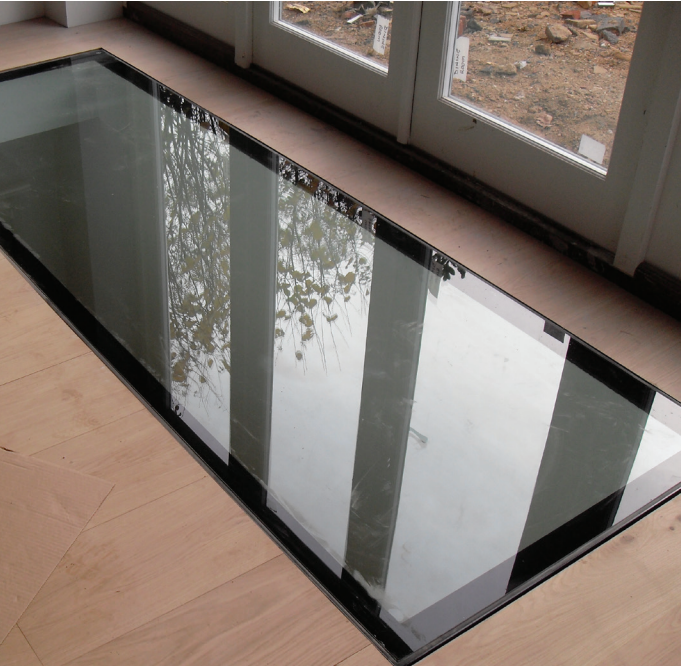
Internal walk-on rooflight
